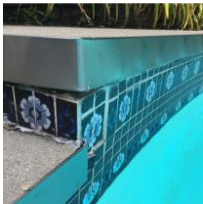
Figure 5:Pushed up coping.
