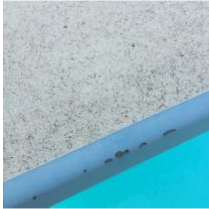
Figure 1:Cracking on the diving board.
