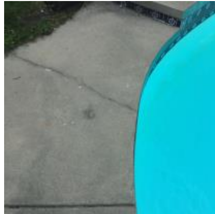
Figure 4:Cracking on the concrete.
