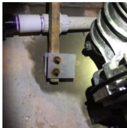
Figure 6:Leaking around the pump.
